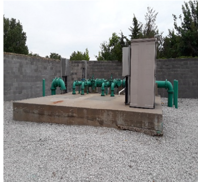
13 Lift Stations Maintained
