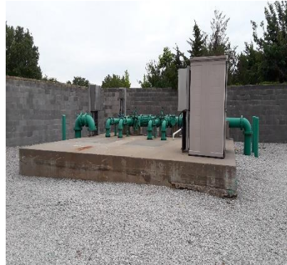
13 Sanitary Lift Stations Maintained
