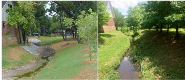
Left: A gabion mattress and turf-reinforcement matting, shown shortly after construction, help protect a garage against stream channel erosion. Right: Fifteen years following construction, the channel's integrity has remained intact
