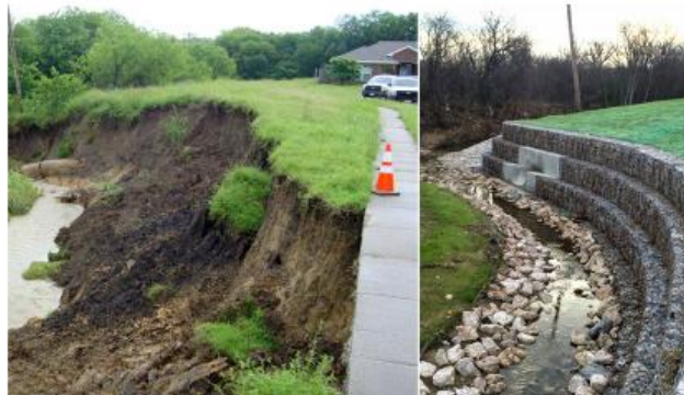
An eroded channel is restored using a gabion wall and rock riprap within the channel.
