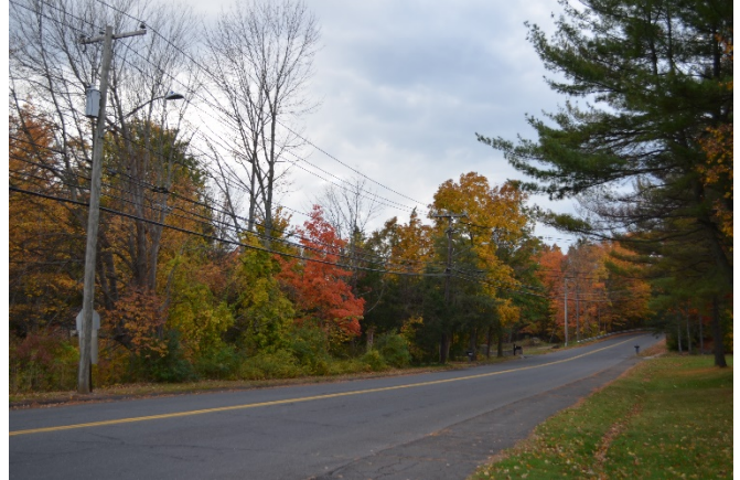
Tanko Lighting's LED Conversion in Berlin, CT
