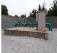
13 Lift Stations Maintained
